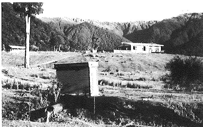
A microhydropower installation in the Southern Alps of the South Island of New Zealand. The intake is in the mountain forest out of the picture to the left. The gross head is 92 m, the flow rate is 16 L/s the electrical output is 3.6 kW which is run by underground cable from the power-house in the foreground to the house on the hill and on to a further house out of sight.
